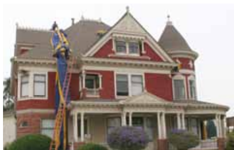
Mission City Fumigation begins tarping the historic Tuttle Mansion. The steep roof and elaborate facade posed quite a challenge.
